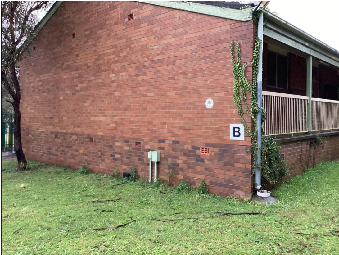
Image 3: Building B (General Learning Building) located in the north west portion of the Site reported on the asbestos register to contain ACM (taken 05/07/2022)
