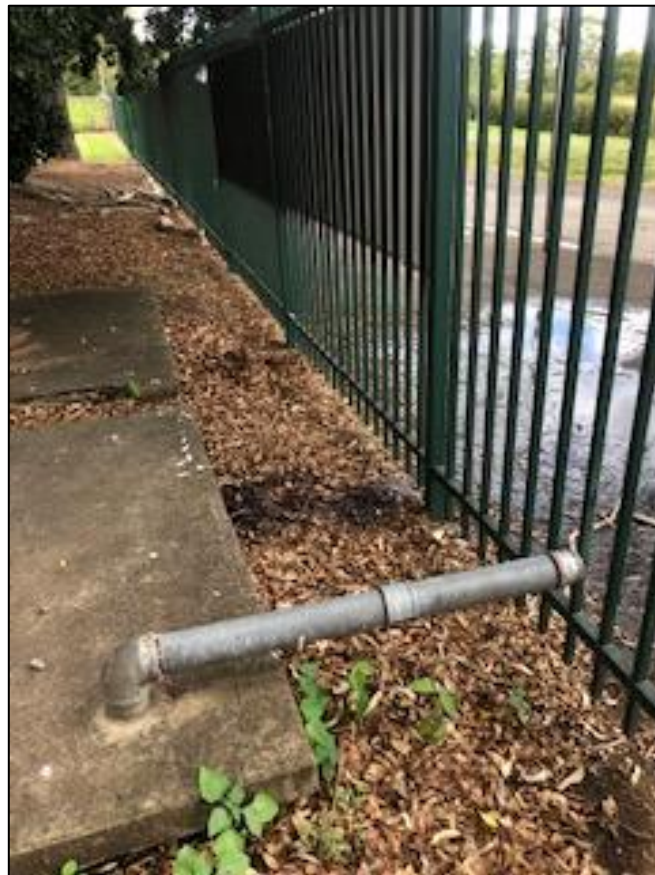
Image 42: Overflow of septic tank near HA09 (taken 13/04/2023)
